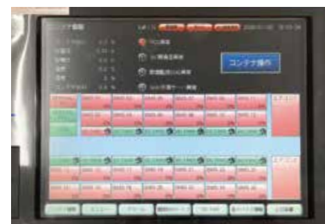
Master Battery Management Unit (MBMU) monitor screen The monitor display is used to monitor and manage the storage battery system that reuses in-vehicle batteries as a “group.”
