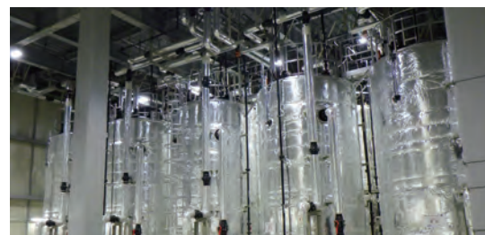
Floor 1: Tank, Pump and PCS
