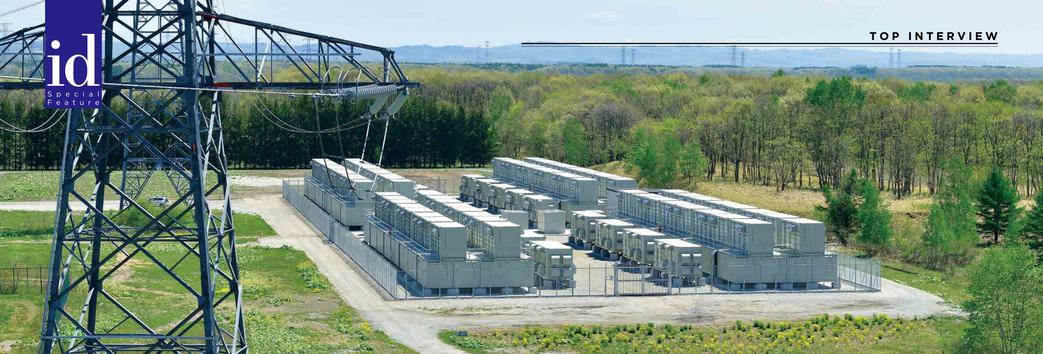
The vanadium redox flow battery delivered to the Minami Hayakita Substation of Hokkaido Electric Power Network, Inc.
