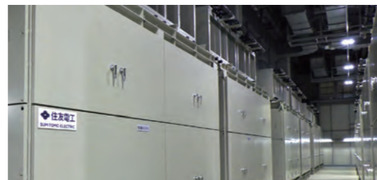
Floor 2: Cell stack and heat exchanger
