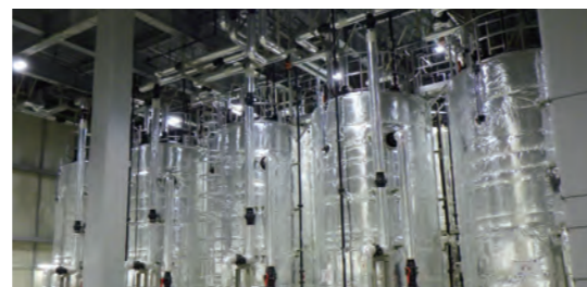
Floor 1: Tank, Pump and PCS
