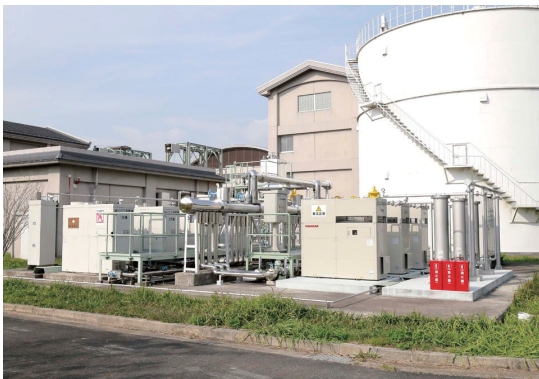
Photo 1. Equipment of power generation using digester gas at Kizugawa-joryu Purification Center
