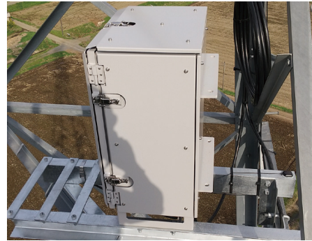
Photo 3. Appearance of the integrator
