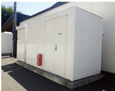
Photo 2. In-house stationary storage battery used for verification
