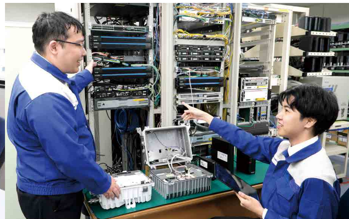
Inspection in the CATV Systems Department
