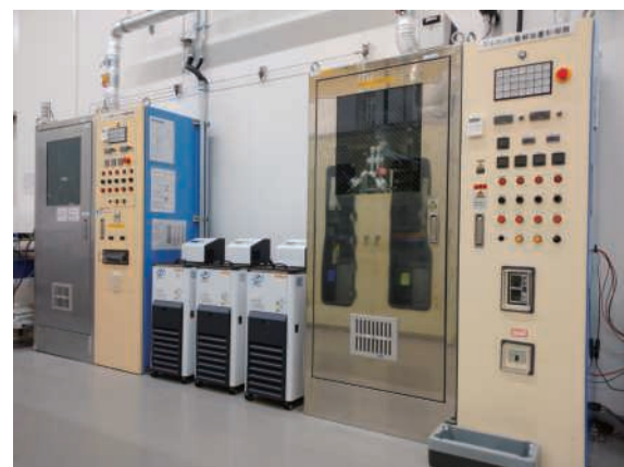
Water electrolysis performance evaluation equipment
