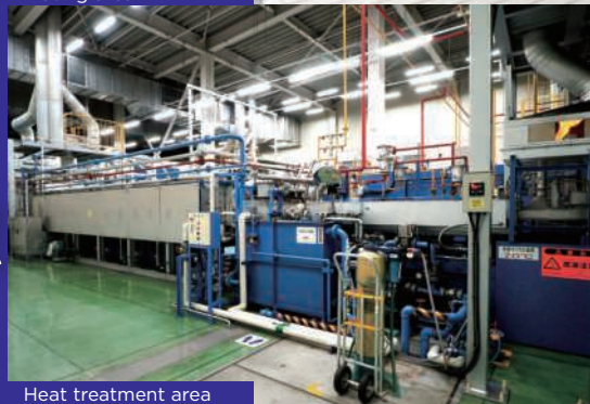
Heat treatment area
