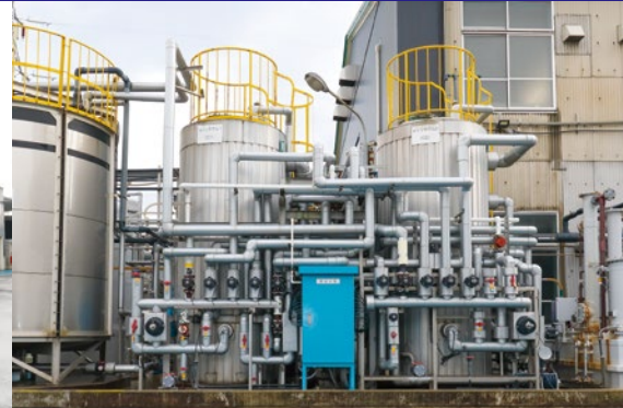
Ion exchange building
