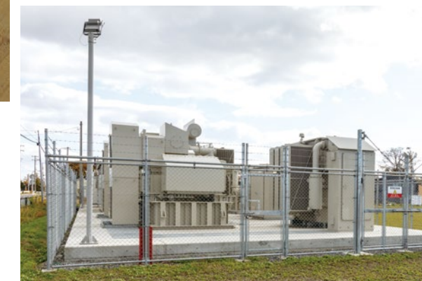
Grid connection switching station
