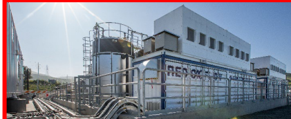
San Diego Gas & Electric (SDGE) 8MWh Wholesale Market
