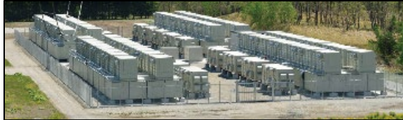
Hokkaido Electric Power (HEP) 51MWh Grid Balancing (wind)
