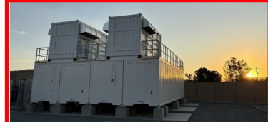
SDGE 4MWh Wholesale Market, Microgrid
