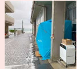
WOTA BOX installed in Suzu City
