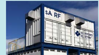
Redox Flow Battery Systems
