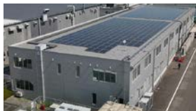
Solar power plant at Sumitomo Electric Printed Circuits, Inc. (Shiga)
