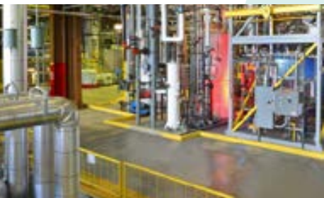
Plant in NY, U.S.A. with recycling system
