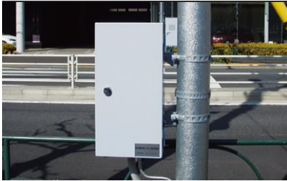
Traffic signal controller
