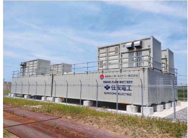
Photo 1. External view of RF battery
