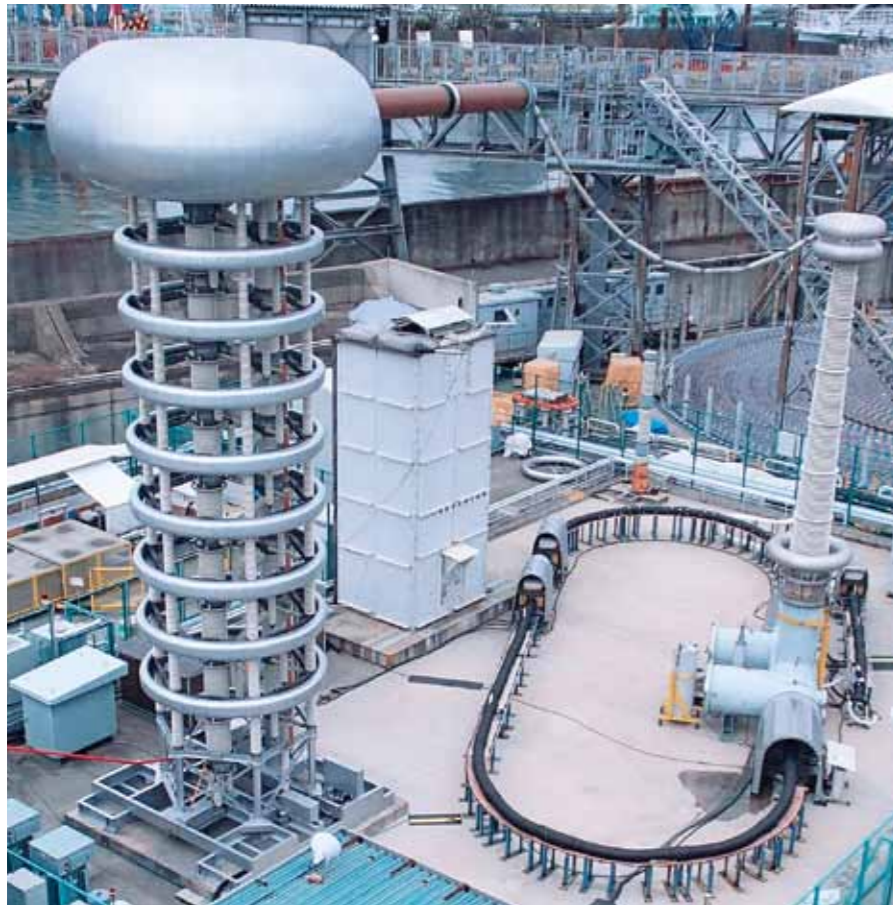
Electrical test laboratory at SEI's factory
