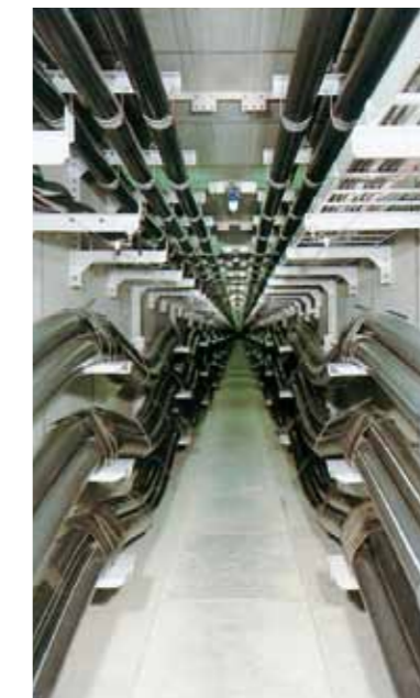
Vertical snaking for EHV XLPE cable in tunnel
