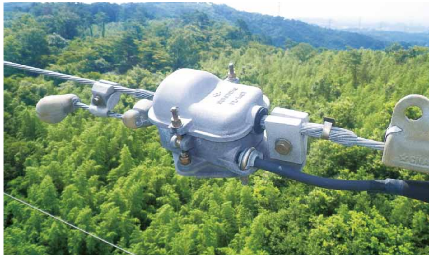
CT (Current Transformer) Sensor for Fault Locating System
