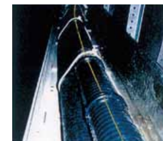
Cable temperature monitoring by Fiber-Optic Sensor
