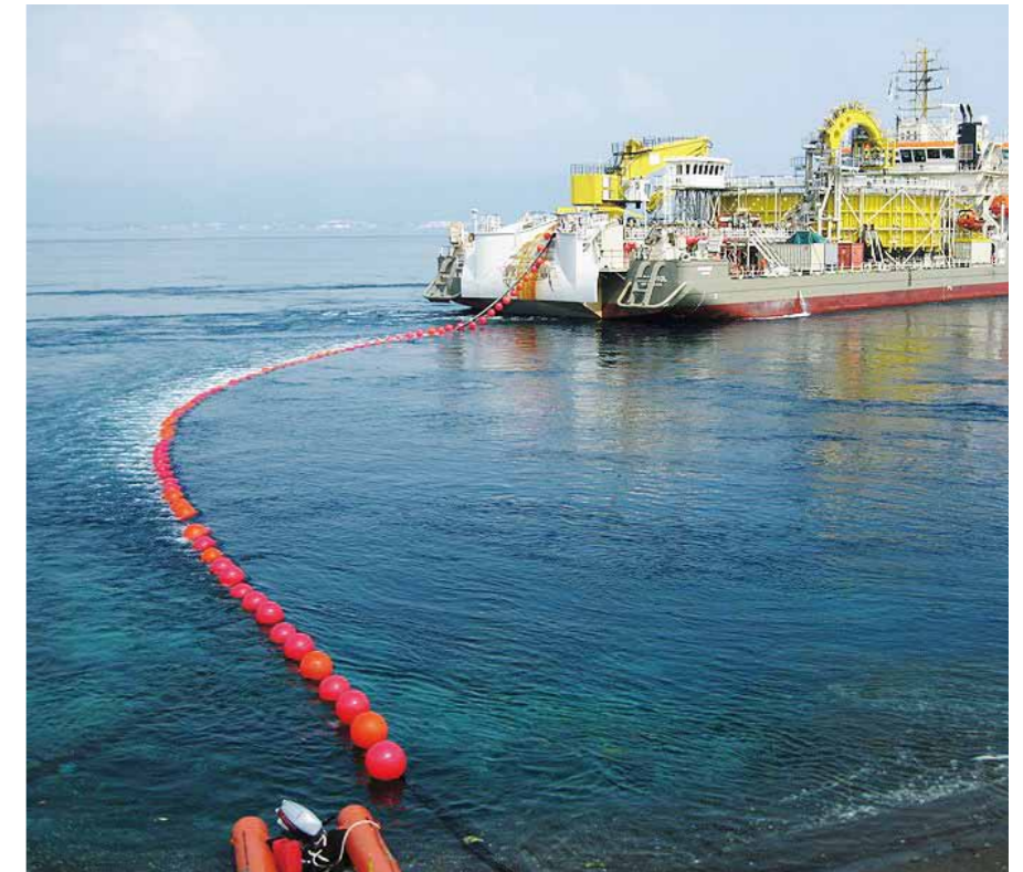
Submarine cable installation under high tidal current by DP-II vessel "Ndurance" in Bali Strait (by courtesy of VBMS)
