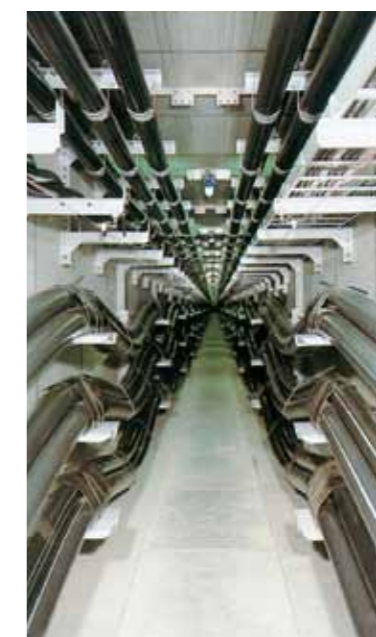
Vertical snaking for EHV XLPE cable in tunnel
