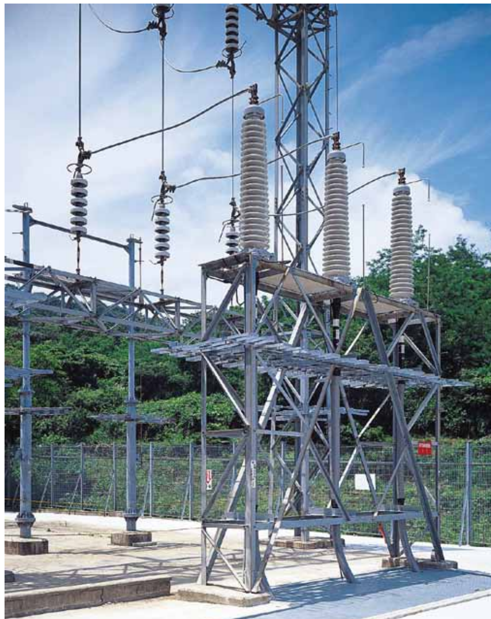
Installed outdoor sealing end
