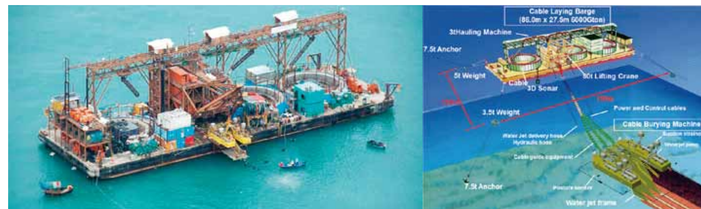
Three cable simultaneous laying and embedding by water jet plow in Hong Kong
