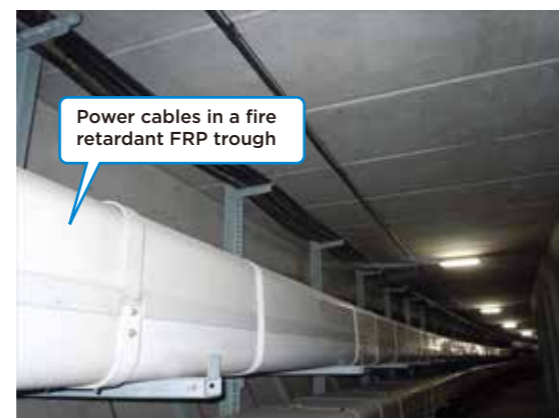
Tunnel for Power Cables
