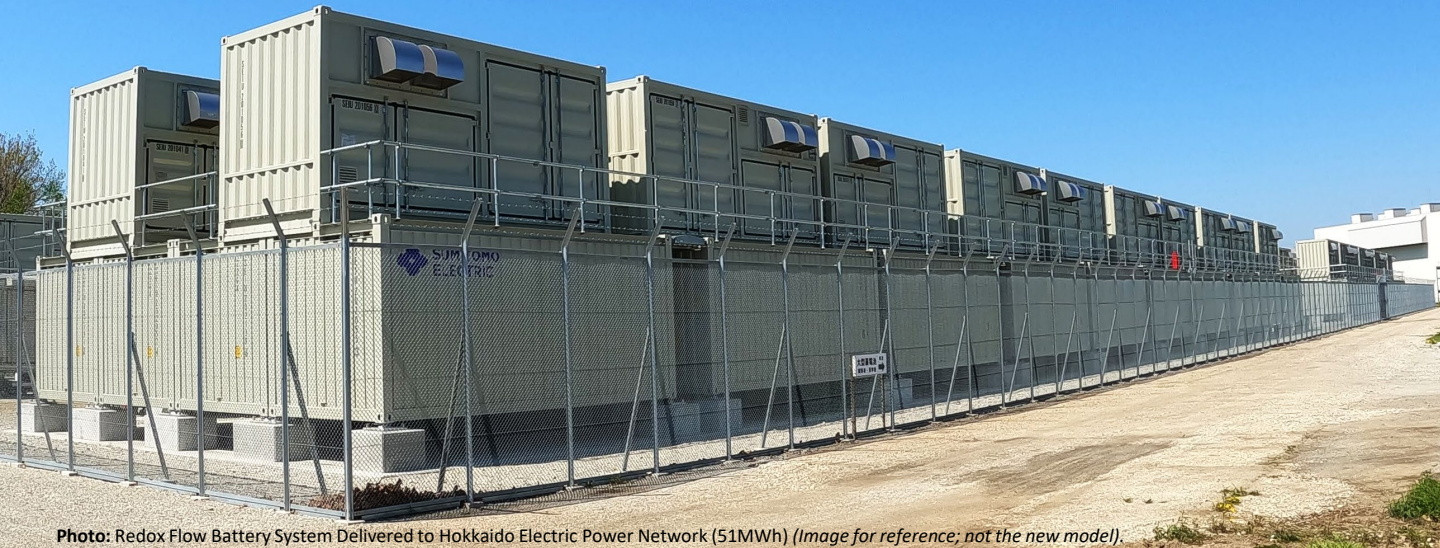
Photo: Redox Flow Battery System Delivered to Hokkaido Electric Power Network (51MWh) (Image for reference; not the new model).
