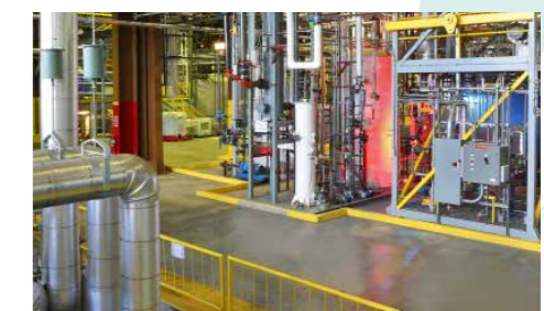
Plant in NY, U.S.A. with recycling system
