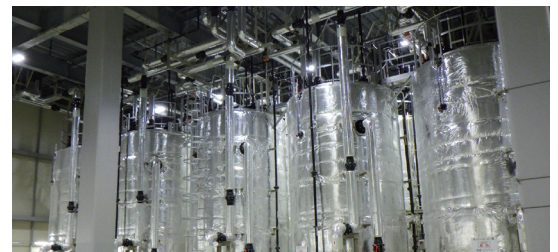
Floor 1: Tank, Pump and PCS
