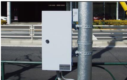
Traffic signal controller
