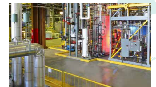
Plant in NY, U.S.A. with recycling system
