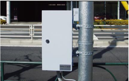
Traffic signal controller
