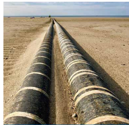
Submarine cable between the United Kingdom
