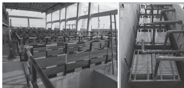
Photo 5. Membrane unit of urban sewage treatment plant in China
