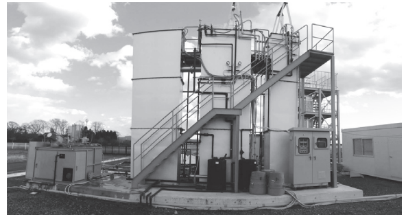
Photo 2. Demonstration Plant jointly with the Japan Sewage Works Agency and Maezawa Industries, Inc.
