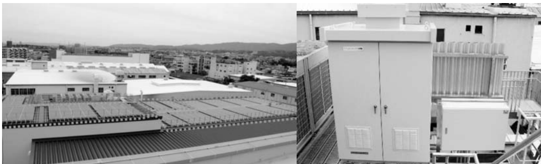
Photo 2. A 100 kW + 10 kW solar power plant installed on the premises of Nissin Electric
