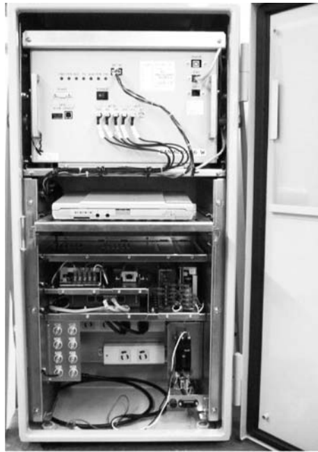
Photo 1. Exterior of radio unit
