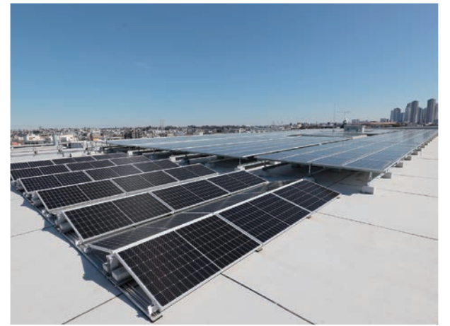
Photovoltaic power generation system constructed on the roof of a training facility "Sumitomo Densetsu Kawasaki Technical Center," which was opened in March 2023
