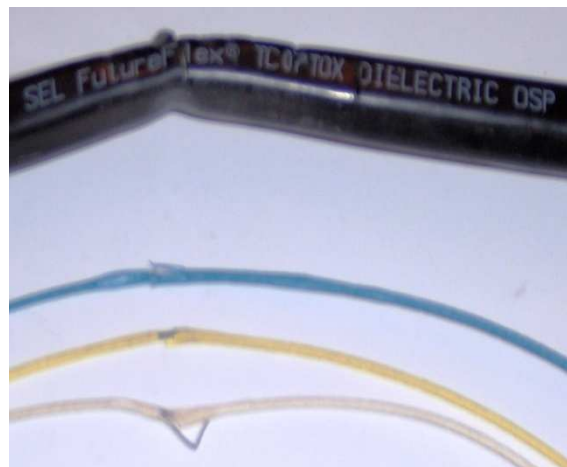
Figure 3 Jacket Cut and Fiber Bundles Damaged
